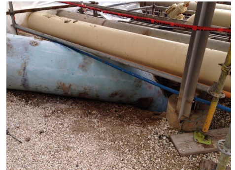
Access point for CIPP liner underneath pipe rack.
