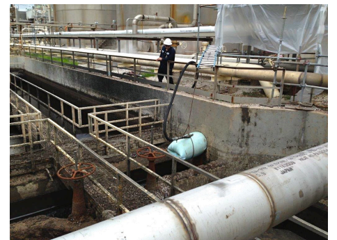
CIPP liner termination point.
