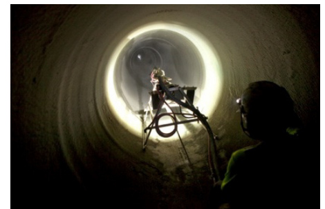
The EcoCast system was lowered into the deteriorated 320 ft. line from a man-way and relined with a structural and corrosion resistant geopolymer.
