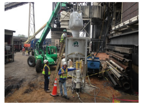
A 54" cooling line, lying beneath IPR Industrial Services EcoCast crew, was leaking into a 13,500 kV room shown on the right side of this photo.
