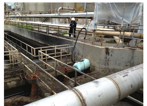
CIPP liner termination point.
