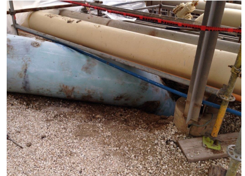
Access point for CIPP liner underneath pipe rack.
